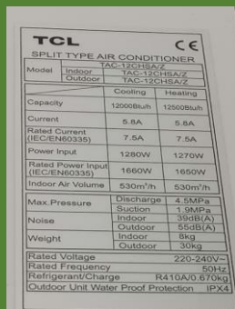
Figure 6: Nameplate of HVAC units installed in experiment bungalows
